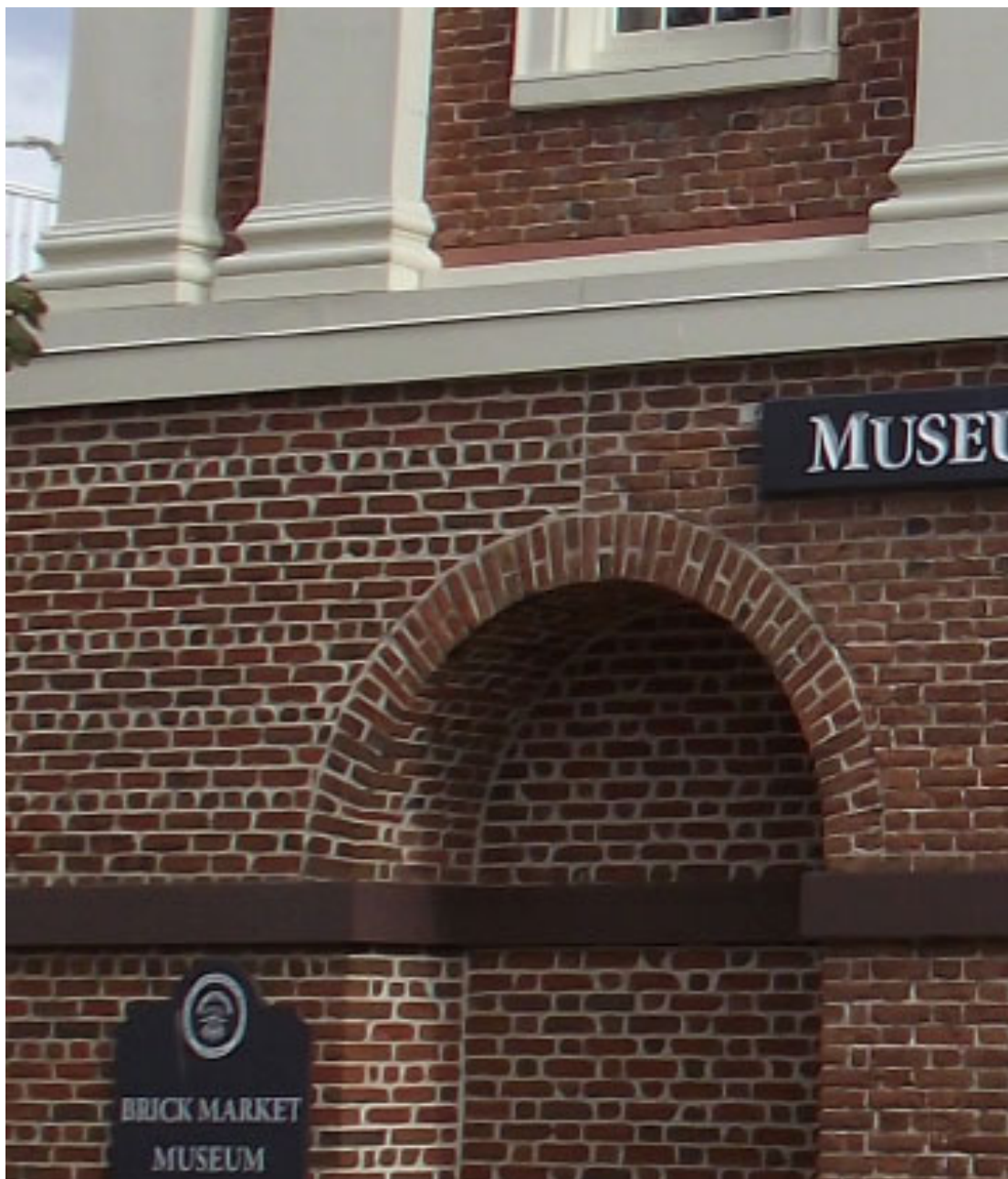
Fig. 17 The Brick Market, Newport, RI (1762 – 1772), Peter Harrison, architect Northwest end of the building, showing change in brick patterning beginning at the top of the arch after 1928 repairs. Photographed by author.
