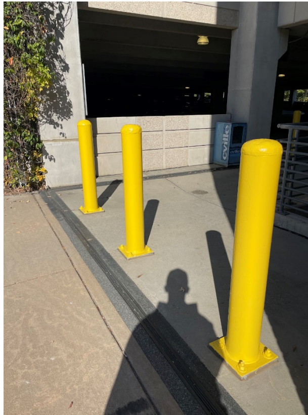
Fig. 2.7.1. Bollard posts located at Culbreth Parking Garage at UVA
