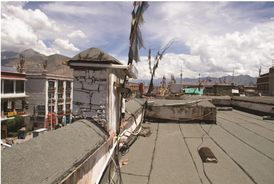
Figure 4.10. Yabshi Phunkhang, Modern Tar Roofing Material on Traditional Roof. August, 2016.
