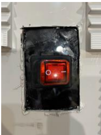
Fig. 23: Electronic box switch
