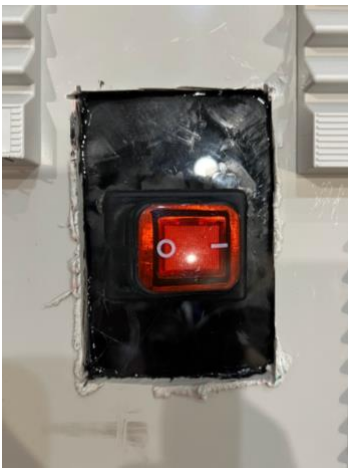
Fig. 23: Electronic box switch
