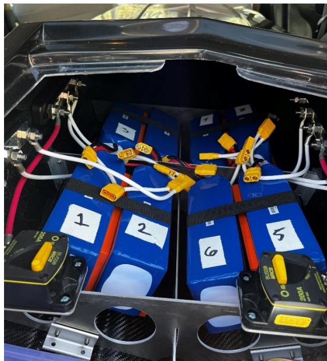
Figure 21: View of the Batteries and Fuses in Position
