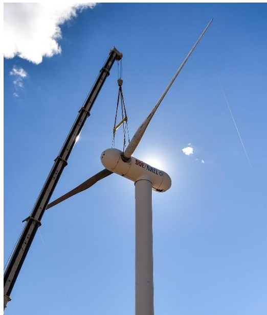
Figure 3-2. SUMR-D rotor being installed on CART-2 at the NREL Flatirons Campus outside Boulder, Co. (photo courtesy of Lee Jay Fingersh, NREL).
