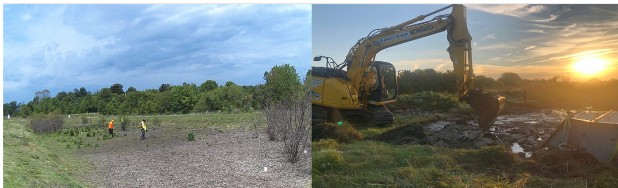
Figure 4.1 Maintenance event in Bioretention (Left: Regular maintenance activity in April 2021; Right: Forebay Restoration in Fall 2021)
