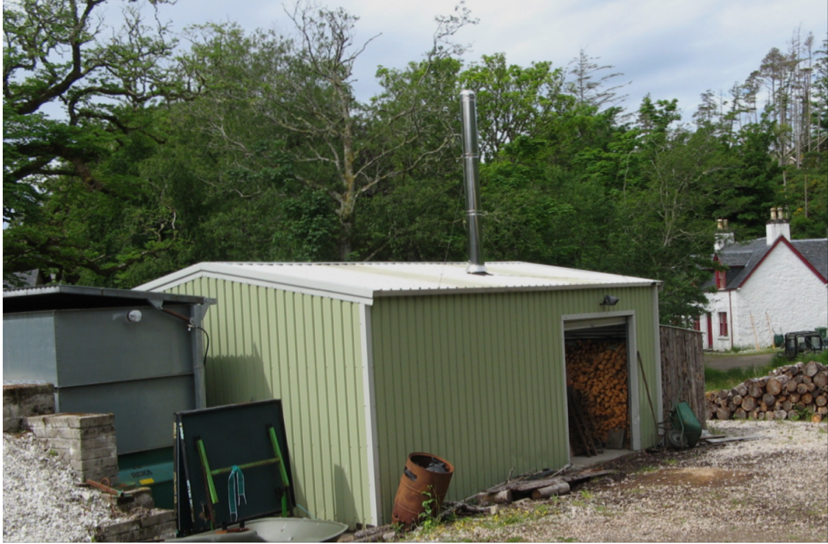
Unused wood chip boiler behind the Glencanisp Lodge in June of 2016.
