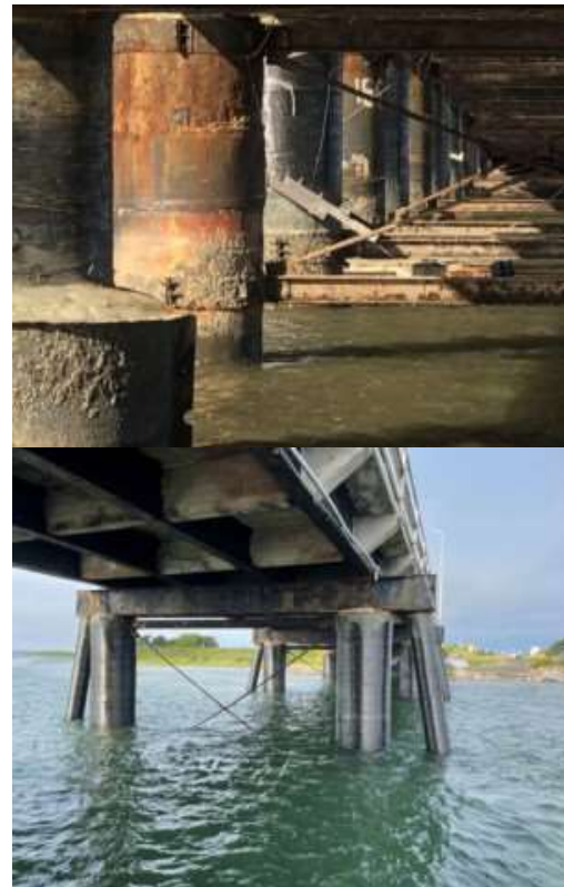
Figure 1: Restored Bridges. The top image illustrates the destructive effects of marine environment, and the bottom image depicts the restored deteriorated concrete with carbon fiber fabric (Adapted by Joshua Garrison (2022) from Underwater Construction Corporation 2022).
