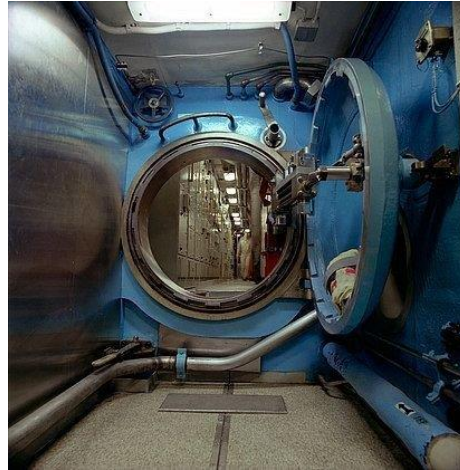
Figure 2: Image of Submarine Watertight Door.
