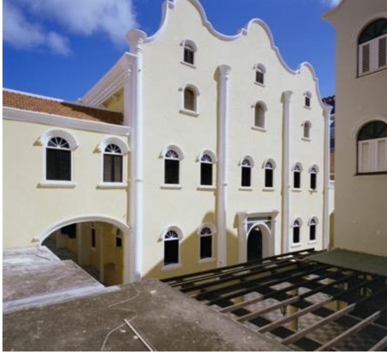
Image 5.7: Mikveh Israel Synagogue, West Facade. Photograph 1994/1995. Cultural Heritage Agency, Amersfoort; Document Number 900,376
