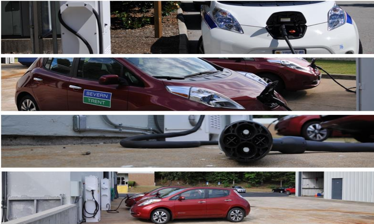
Figure 7. Advanced bidirectional fast charger to reduce utility costs with vehicle-to-grid (V2G) and demand charge management integrated into logistics systems (Source: Fermata LLC 2017)
