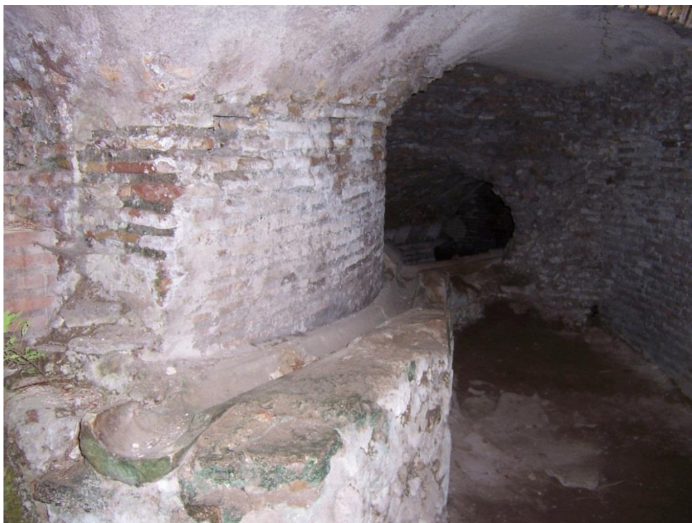
Figure 3-35: Small Drainage Channel in the Substructures of the Terme del Foro
