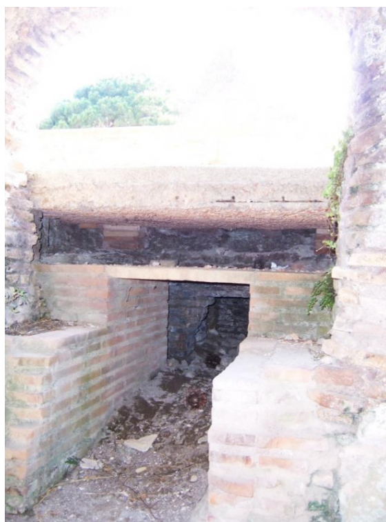
Figure 3-164: Furnace Opening for Pool \beta in Room 19 showing Damage to Floor and Walls
