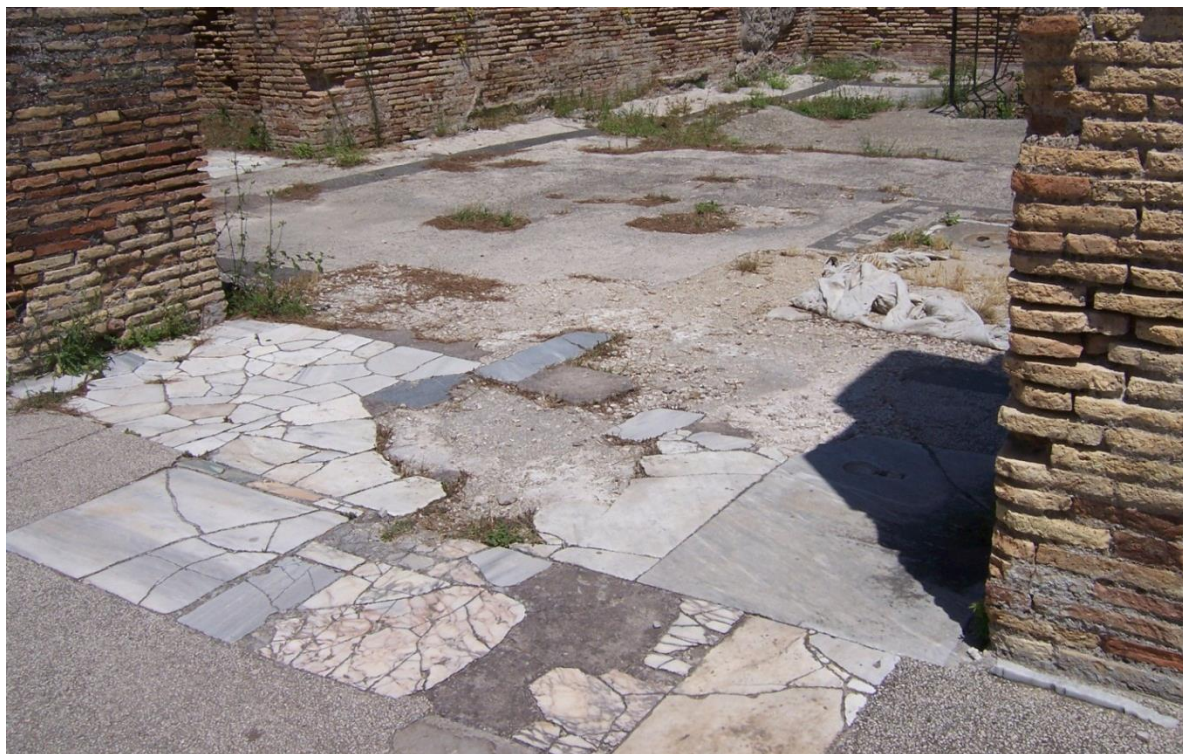
Figure 4-16: Threshold of Door O showing Fragmentary/Dissimilar Pavement Composition
