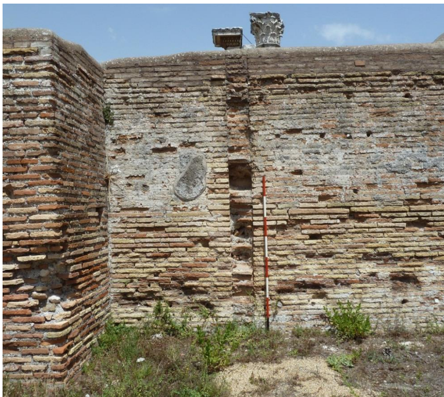
Figure 3-74: Fistulae Slot in Wall k in Room 2
