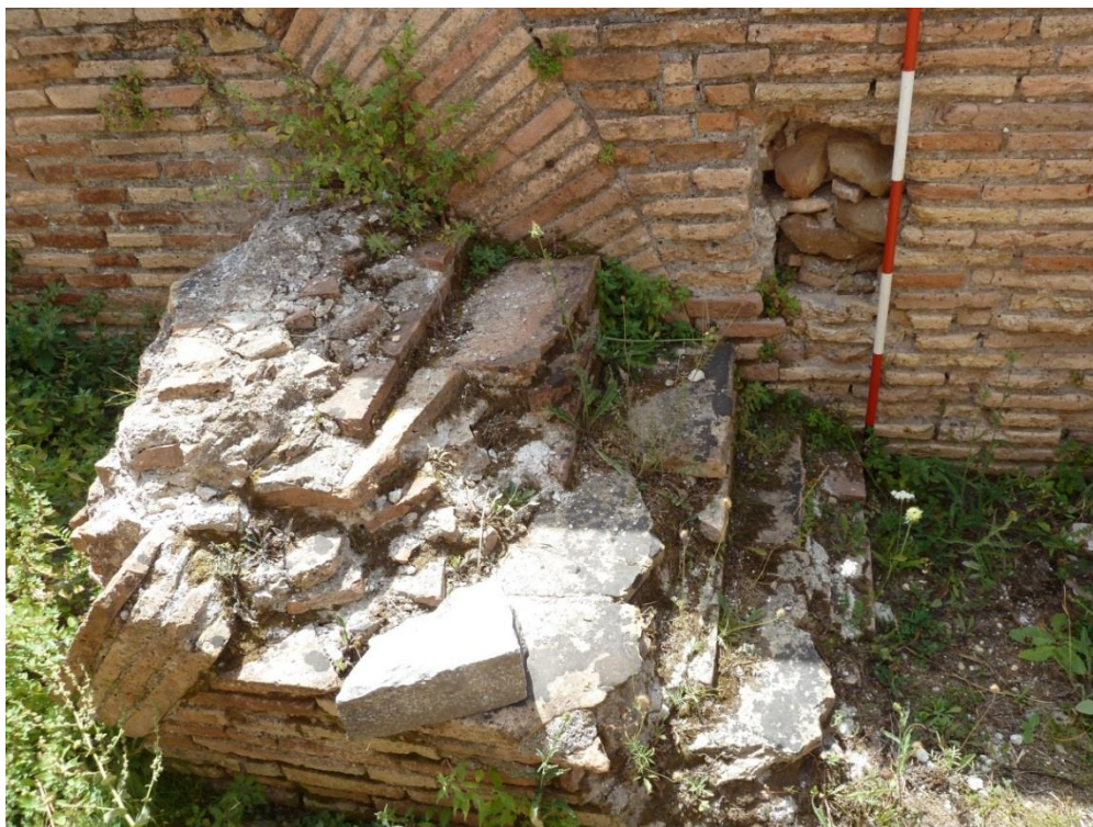
Figure 3-43: Staircase in Room a2 Possibly Leading to Upper Stories of Room a
