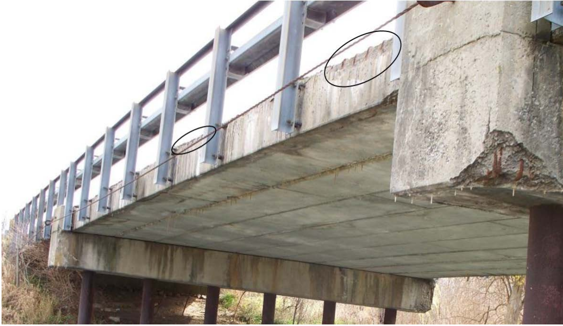
Figure 43 - Existing damage on the Center Span's Beam 1 (Steinberg, 2011)
