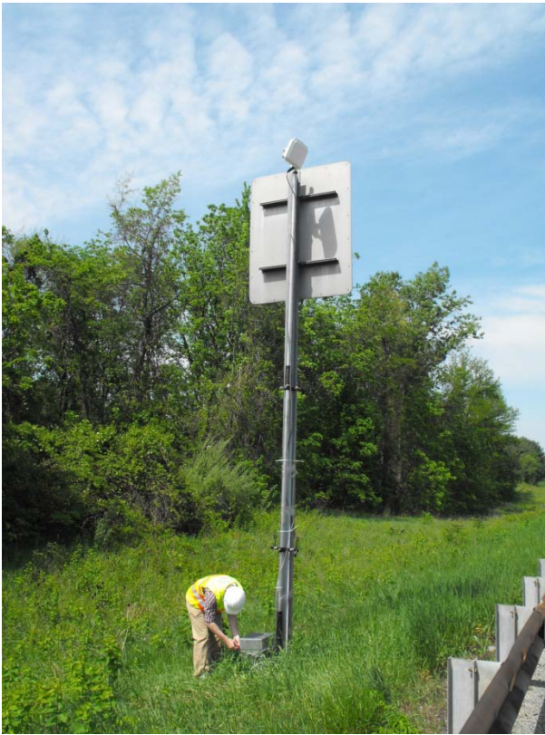
Figure 10. Setup of Wavetronix device along side of I-81.
