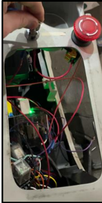
Fig. 15. Emergency stop inputs: autonomy switch (left), E-stop button (right)
