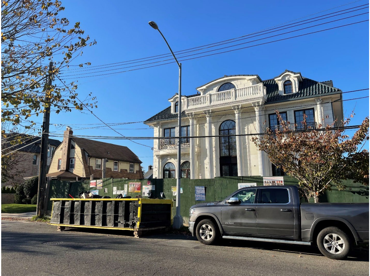
Figure 4-4 McMansion under construction in the Cord Meyer tract dwarfing the older house to the left (personal photo).
