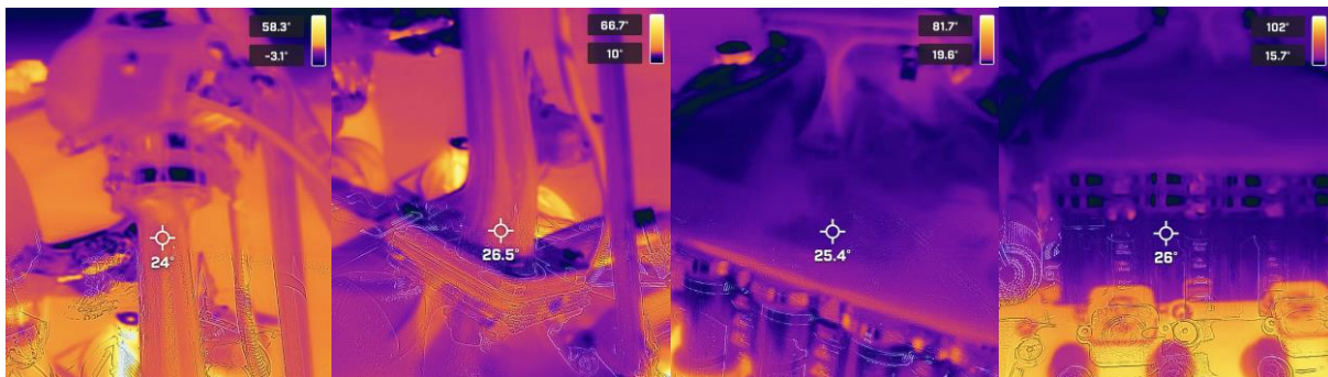
Figure 9. Thermal camera captures (in °C) of intake components
